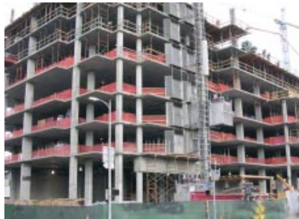
EVO, one of Howard S. Wright's top projects, is a high-profile condo project in Los Angeles.
