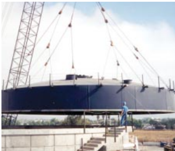
Carl Overaa & Co. is working on the Dublin-San Ramon Wastewater Treatment Plant.
